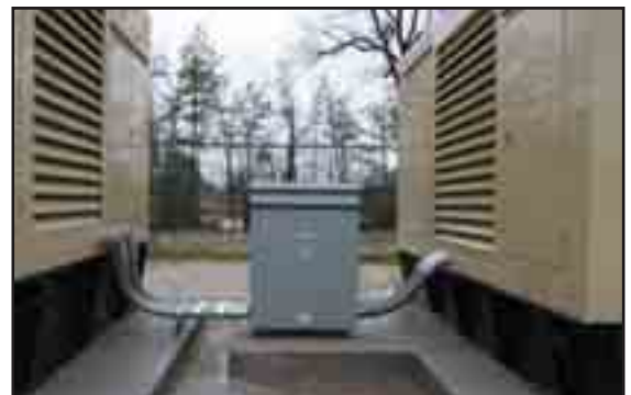
Figure 9: Photo of multiple winding reactor installation.
