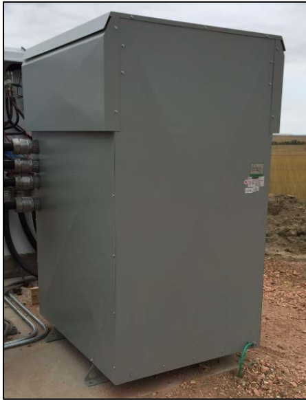
Fig. 4 1100 HP INVERSINE AUSF Sinewave Filter Installation
