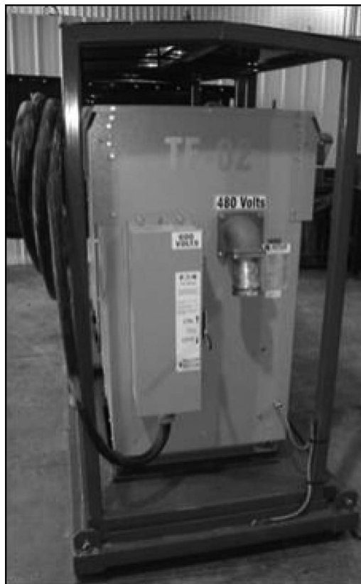
Fig. 21. Wide-spectrum harmonic filter fit for drilling rig application.
